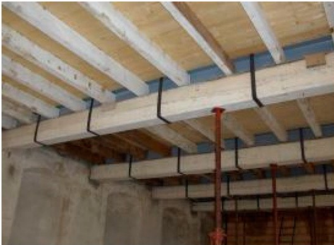
Figure 11. Reinforcement of a timber beam using a stainless steel H-shaped beam applied on the compressed area.
